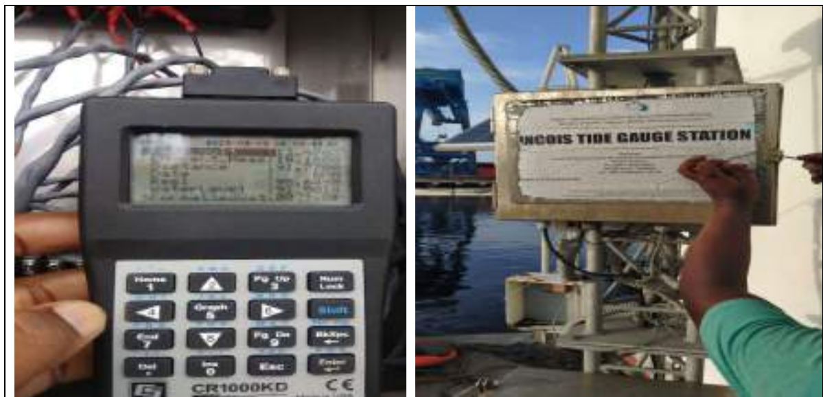
Automatic Tide Gauge Monitoring System
