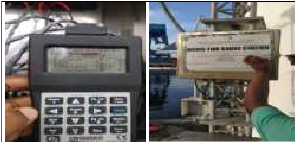
Automatic Tide Gauge Monitoring System
